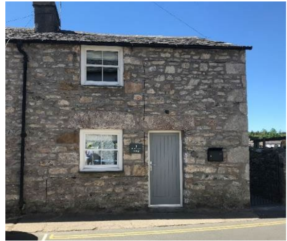
Figure 5. End cottage, the Causeway in 2019. Both the windows and door have been removed and replaced under permitted development, eroding the character of the terrace.
