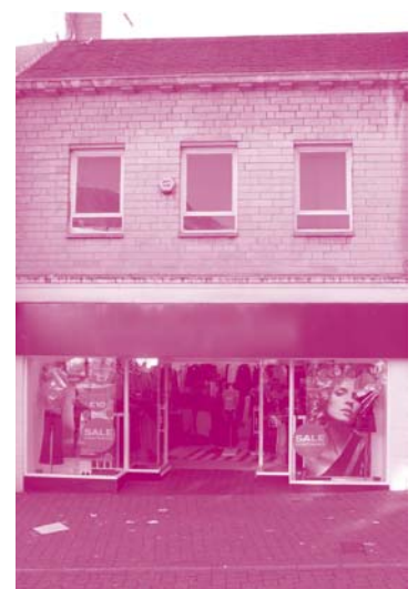
A shopfront without much by way of framing, which therefore provides little apparent support for the masonry that appears to float above
